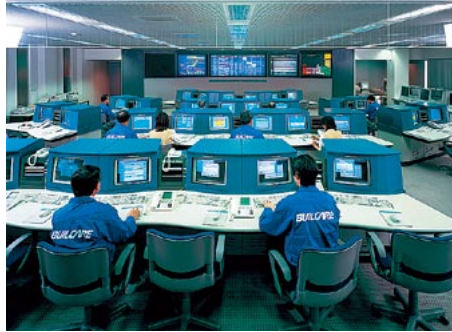
Customer Center, Hitachi Building Systems Co., Ltd. Monitoring elevators and other building equipment
