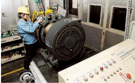
Inspection of elevator machinery, Hitachi Building Systems Co., Ltd. All elevators are subject to rigorous inspections for vibration and noise. Only products that pass these tough inspections are shipped.
